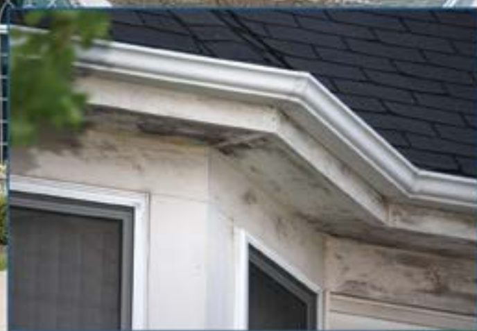
Wood Soffits require cleaning, scraping and painting
